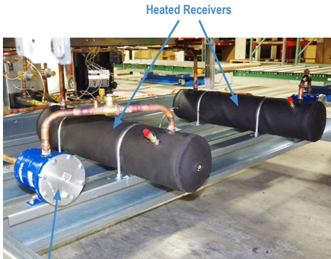
Installed - Heated Receivers
