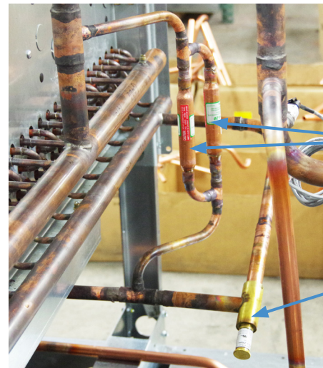
Installed - Head Pressure Control Valve (adjustable for larger chillers)
