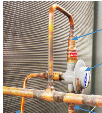
Installed - Head Pressure Control Valve (non-adjustable for smaller chillers)
