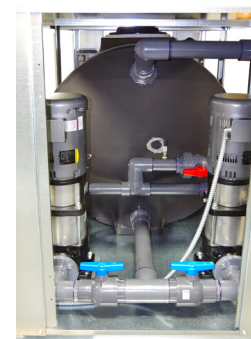
Inside View: Model: RRT600H, Dual Vertical 10 HP Process Pumps
