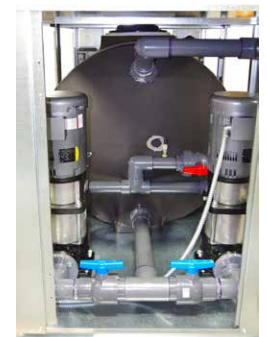
Inside View: Model: RRT600H, Dual Vertical 10 HP Process Pumps
